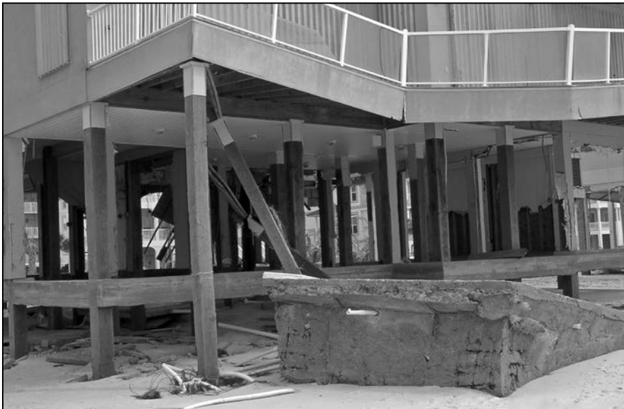
Figure 28: Failure of two piles supporting an elevated deck that was likely caused by movement of a spa
