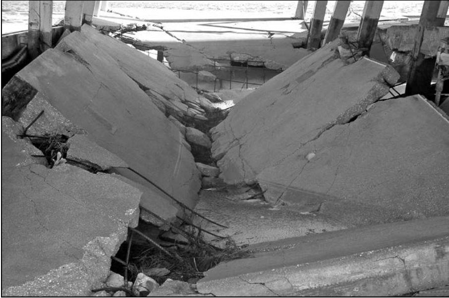
Figure 20: Damage to building foundation caused in part by failure of the reinforced slab undermined by erosion
