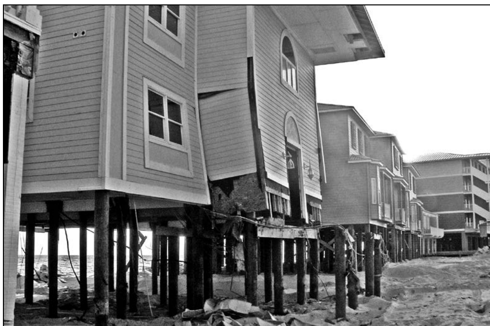
Figure 1: Damage to an elevated building as a result of stairs that not break away cleanly
